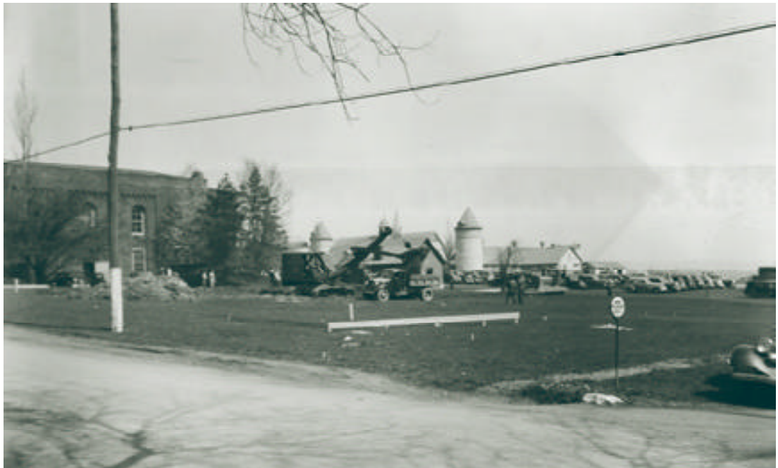
This photo was taken by Dr. Wallace E. White, professor of wood utilization, on April 21, 1938, the first day of Ferguson Building construction when the top soil was stripped from the site. The photo is taken from the south corner. You can see the Stock Judging Pavilion (now the Pavilion Theatre) behind the Ferguson site, a parking lot, and the dairy (where Agricultural Administration Building now stands).
