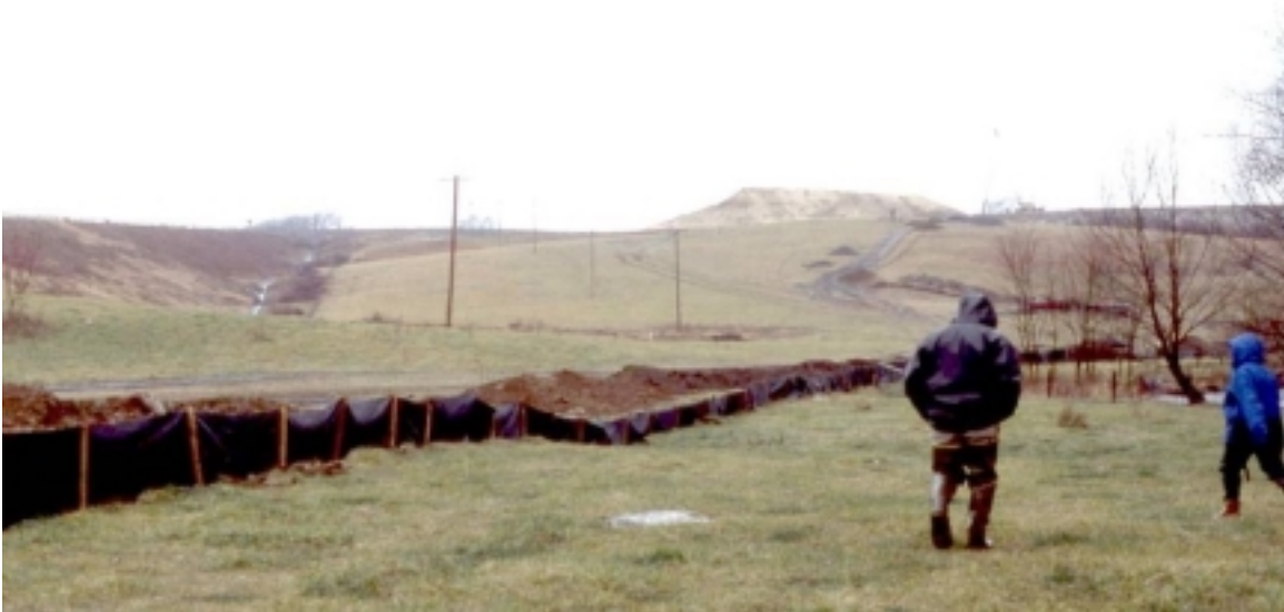
Picture 1. View of construction area soon after installation of silt fence (November 1999) at the Park Avenue site. Notice the large buffer area between future construction on the hill side and the stream (right of person in blue jacket).
