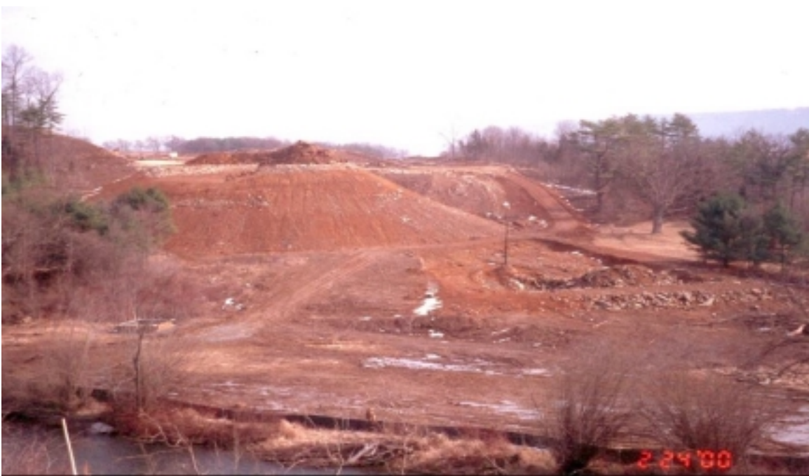
Picture 5. The Rock Road site after the initial land clearing a few months after construction started. Spring Creek can be seen in the lower left of the photo.
