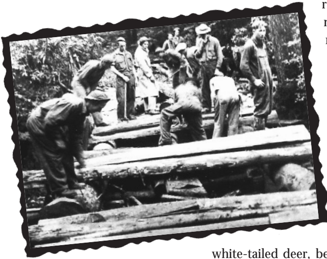
Civilian Conservation Corps workers use chestnut logs to construct a bridge in Shenandoah National Park, Virginia. Courtesy Shenandoah National Park Archives.
