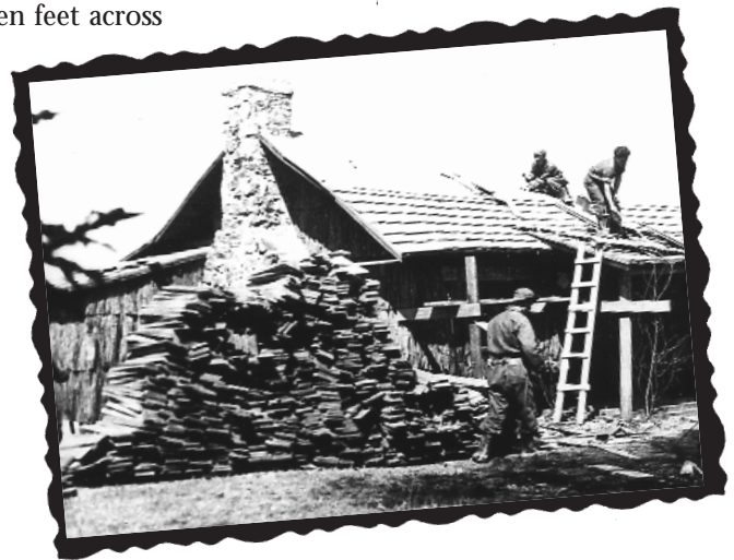
Civilian Conservation Corps workers roof a cabin with chestnut shingles. Courtesy Shenandoah National Park Archives.
